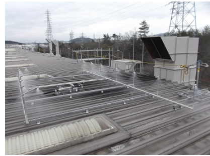
Sprinkler system installed on the factory roof (Osadano Plant)
