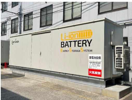
External appearance of the container type power storage system
